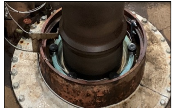
AMPS installed and in operation since April 2021.
